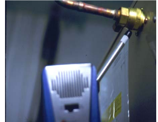
Use HFC Leak Detectors
